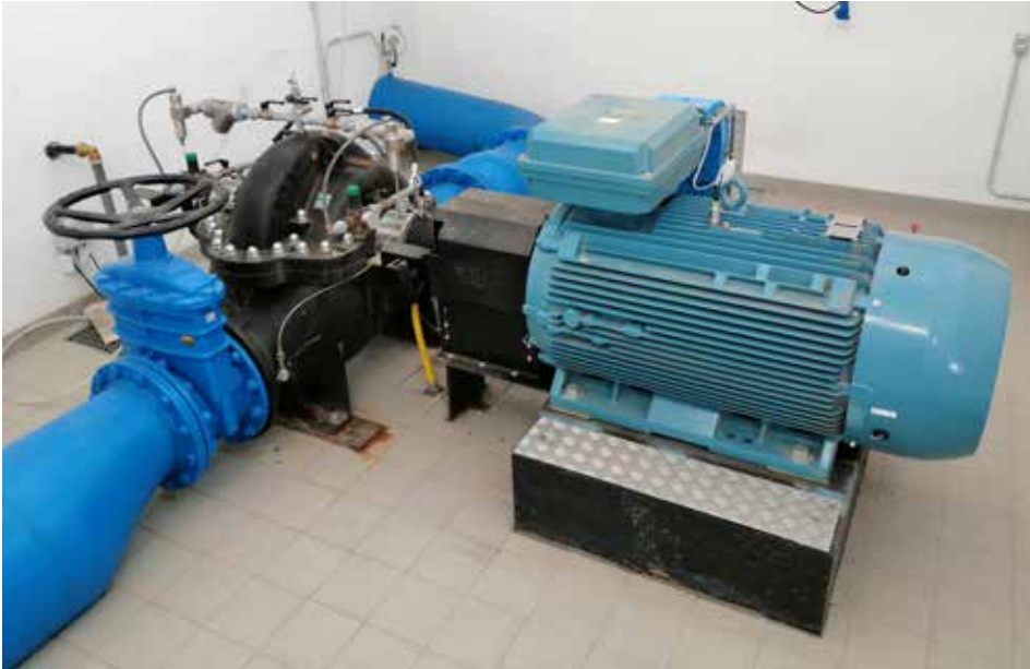
NR. 1 SKDZ-4P 250-560 315kW HIGH EFFICIENCY VERSION WITH PUMP EFFICIENCY > 80% AND ABB IE4 SYNCHRONOUS MOTOR
