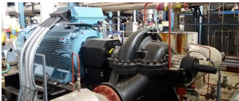
NR. 2 SKDZ-4P 250-750 1000kW SERBIA DISTRICT HEATING
