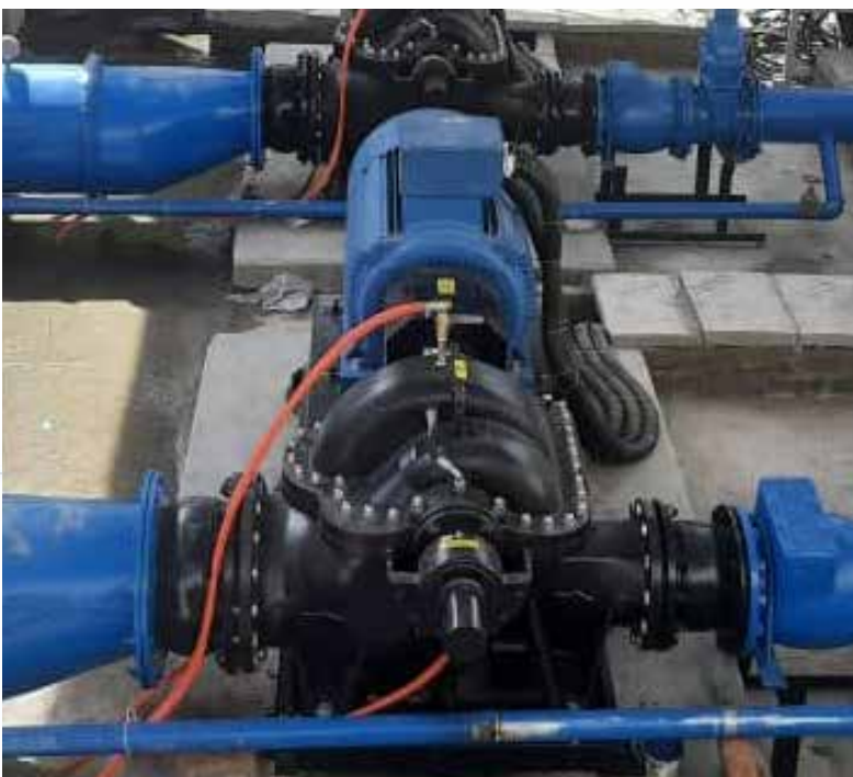
NR. 5 SKDW-4P 250-400 200kW AFGHANISTAN ONE OF THE LARGEST PUMPING STATIONS POWERED BY PHOTOVOLTAIC PANELS IN THE WORLD
