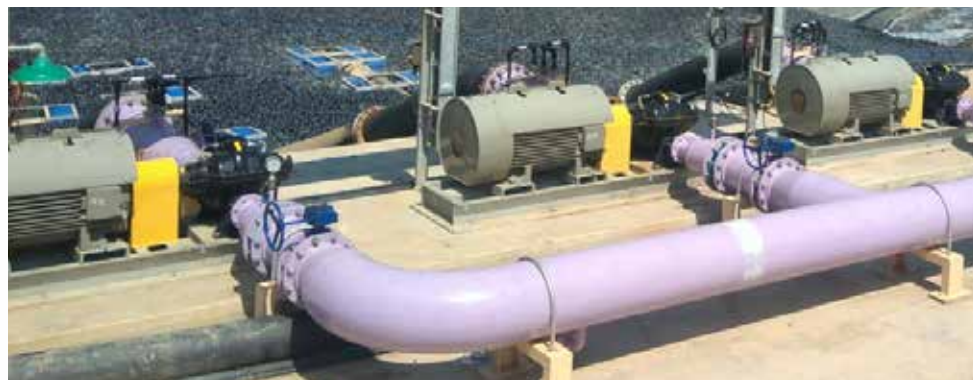
NR. 15 SKD 125-335 AUSTRALIA DEWATERING IN A GOLD MINE
